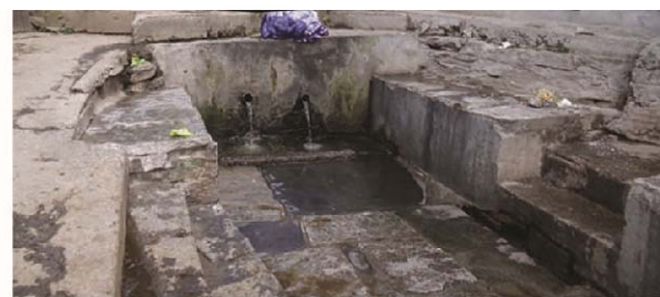
Figure 6: open and insufficient drains
