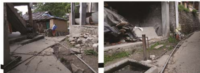
Figure 5: Exposed water supply lines
